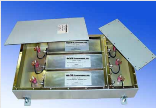
Multi line filters installed in a cabinet
