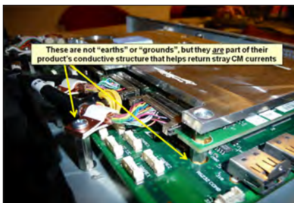
Figure 14. ... and neither are these “earths” or “grounds” for SI, PI or EMI.
